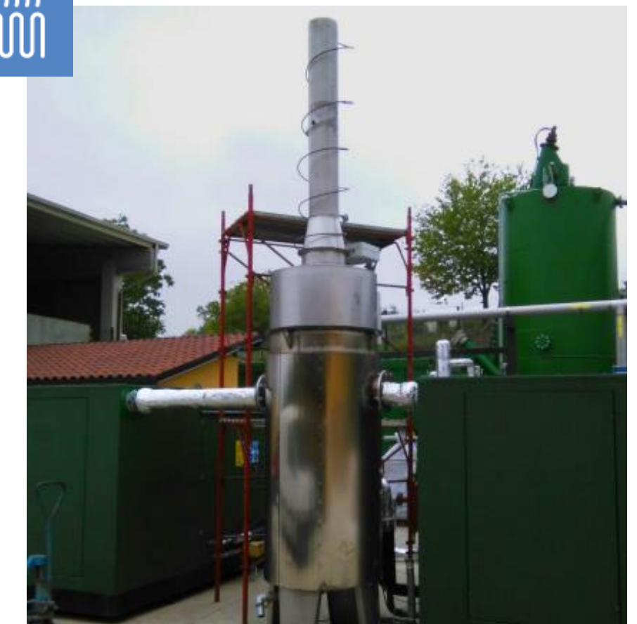
BIOMASS COGENERATION PLANT (ASTI)
